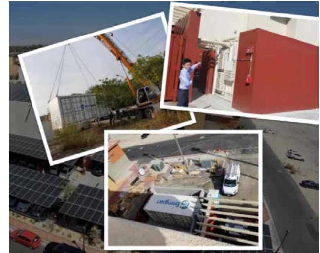
CA, USA, 750kWh, LFP, Utility Grid+PV
