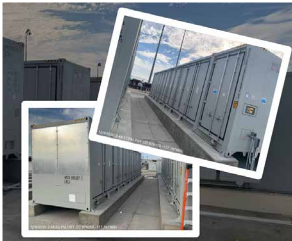
Southern California, USA, 80MWh, LFP, Grid Support
