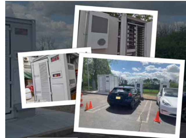
NY, USA, 300kWh, LFP, Energy Buffer
