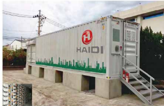
Taiwan, CN, 1MWh, LFP, Peak Shaving
