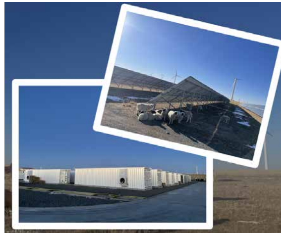
Inner Mongolia, CN, 30MWh, LFP, Wind&Solar Farm
